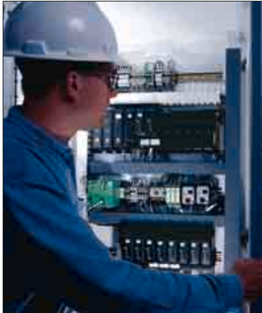
The DeltaV I/O and fieldbus terminators mounted in a remote junction box.
